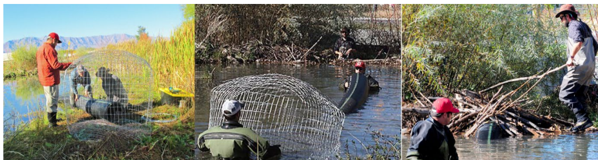
Figure 27: Pond leveler installation. From left: securing flexible pipe in cage to protect inflow from being clogged; placing pipe into beaver pond; rebuilding beaver dam after setting pipe into notched dam at desired water height.
